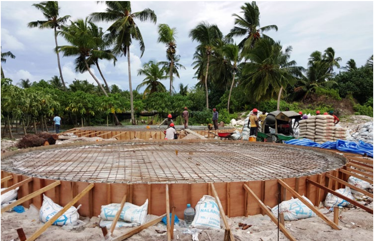
A team of workers building a water tank on Thoddoo island, in Maldives © Ishaq Ashraf, IWRM Project Manager, Ministry of Environment and Energy, Maldives.
