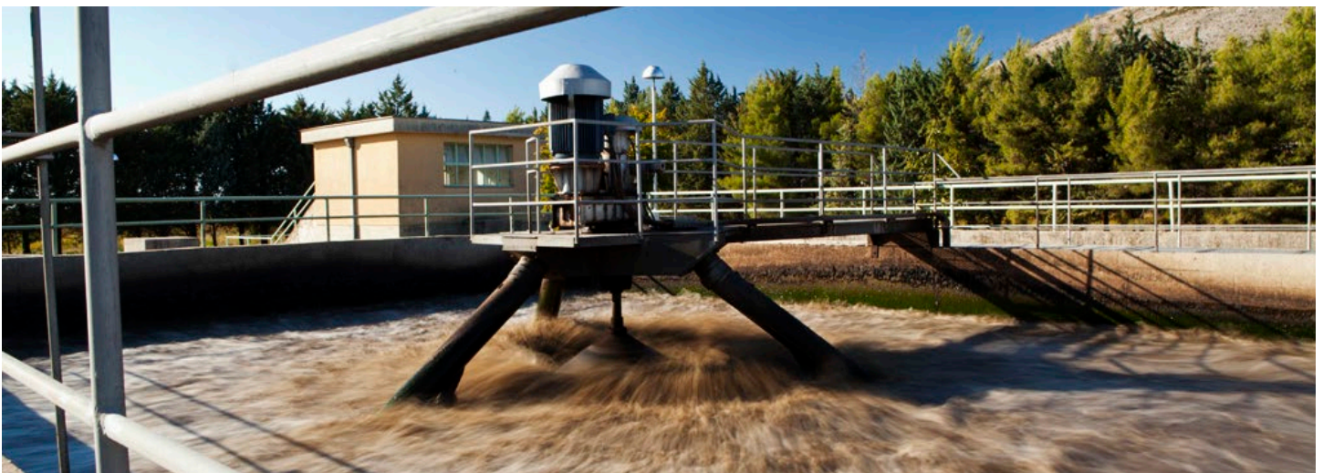
Trebinje Wastewater Utility near Trebinje, Bosnia and Herzegovina. © Max Gudczinski.
