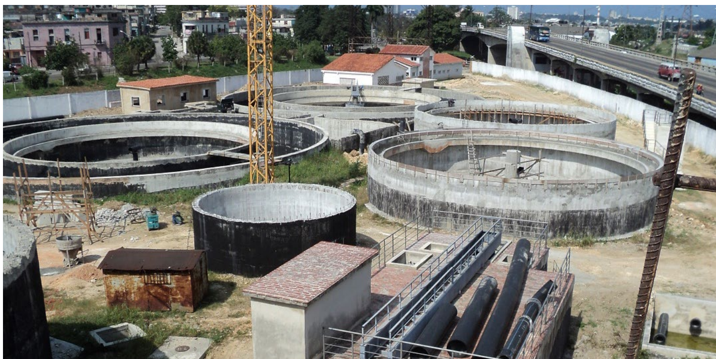
Wastewater Treatment Plant Aerobic Reactor © La Havana Bay Project.
