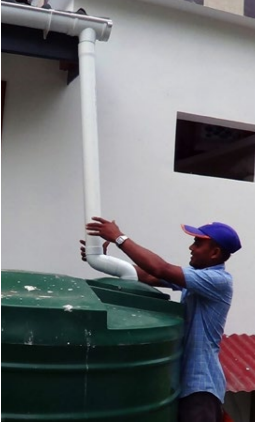
Rain water harvesting installation on the island of La Digue, Seychelles © Sandra Folette, Project Manager, Public Utilities Corporation, Seychelles.
